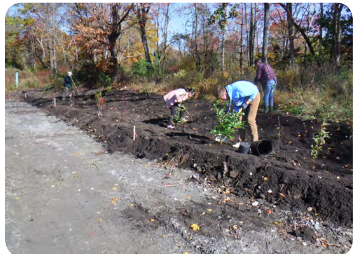
In the top picture is NWCD staff installing a rain garden behind the Bethlehem Town Hall. The bottom two pictures are Taft School volunteers planting a rain garden by the Heminway Municipal Office Building in Watertown
